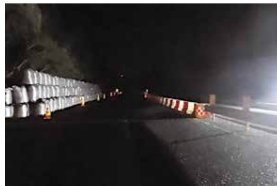
(Emergency recovery work status) Road closures lifted three days after the disaster.
